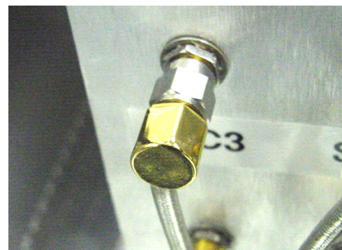
GOLD CAP ON SMA CABLES INSIDE RACK
