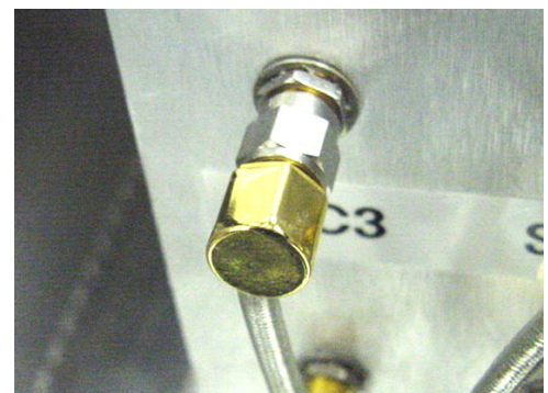
GOLD CAP ON SMA CABLES INSIDE RACK
